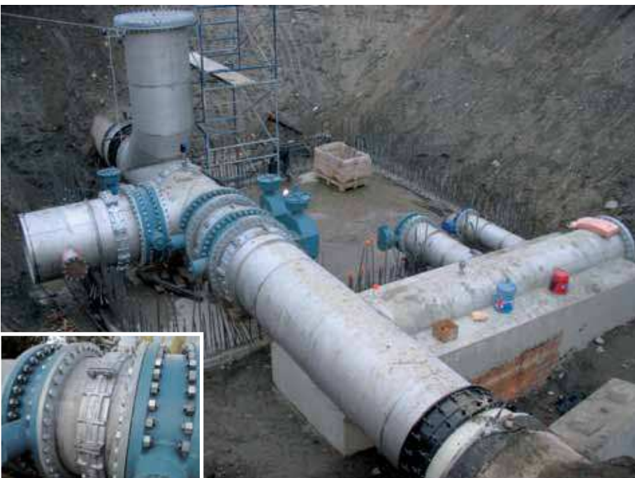
24" (600mm), 36" (900mm) and 48" (1200mm) Model R-88 Couplings with stainless steel rings used on stainless steel hydro electric pipe line, Vernon, British Columbia, Canada
